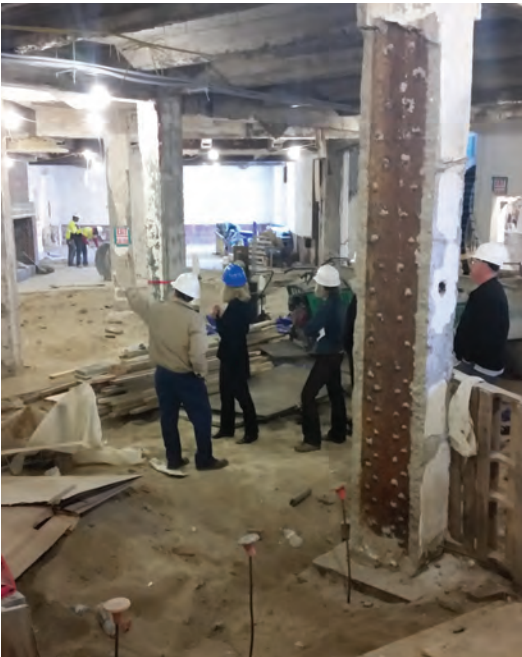
John Hancock, center white helmet explains the extensive renovation of the basement level.
